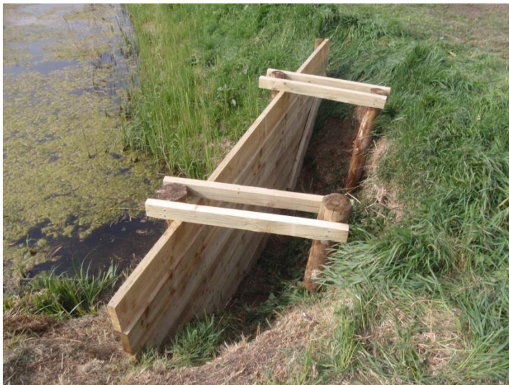
Wood piling before back-filling. Holes drilled in the piling create kingfisher nest sites.
